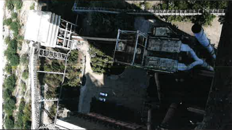
Coal Belt Conveyor
