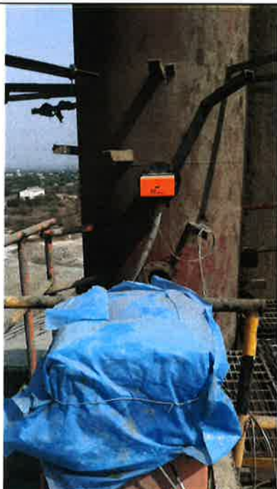
CEMS from Cement Mill - 1 Stack
