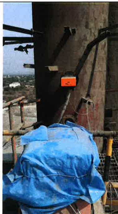
CEMS from Cement Mill - 2 Stack
