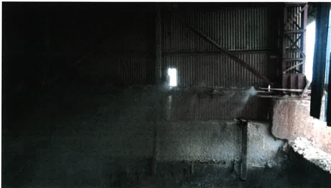
DRY FOG SYSTEM IN LIMESTONE DUMP HOPPER
