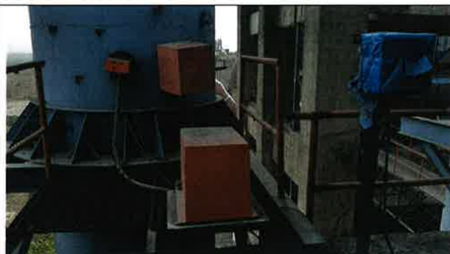
CEMS from Coal Mill Stack
